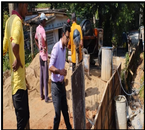
Const. of Concrete Surfacing Road with Retaining wall at Ekkamuthu Lane, Kandy Road, Andankulam.
